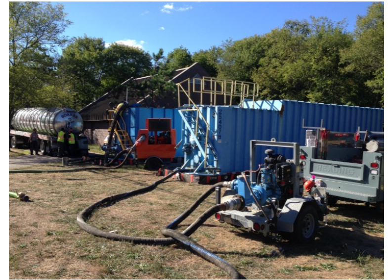
Emergency Response to FM Break
