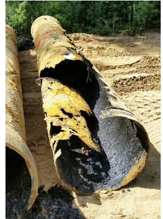
Failed Force Main Section CASE STUDY NO.1
