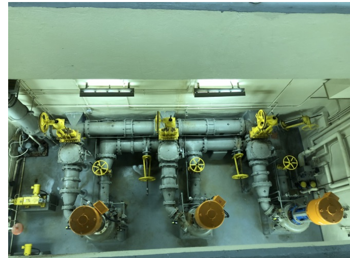
Site Visit to Pump Station CASE STUDY NO.2
